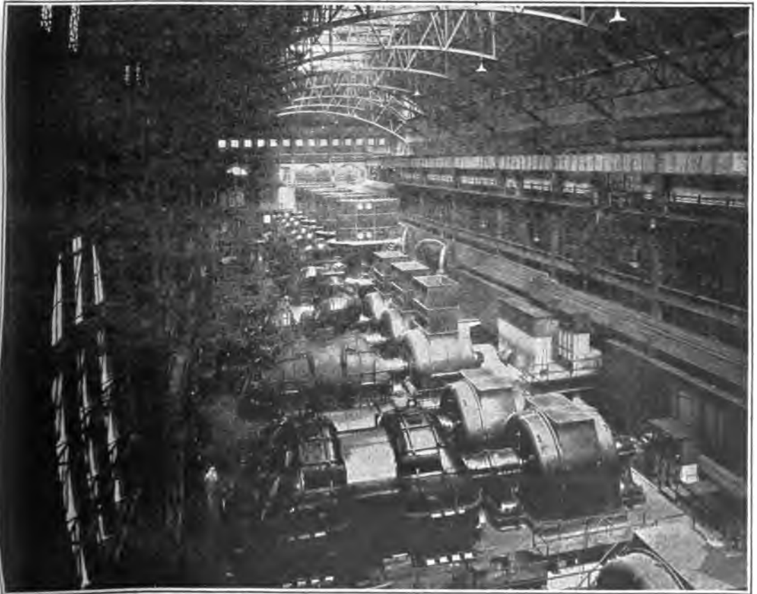
FIG. 1. IN THE FOREGROUND IS A SMALLER DUPLEX TURBINE; JUST BEYOND IS THE 100,000 HORSE-POWER GIANT
